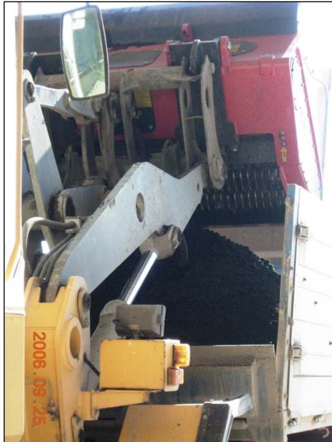
Figure 6. The ALLU at work and the rubber/bitumen mix falls directly onto the lorry.
